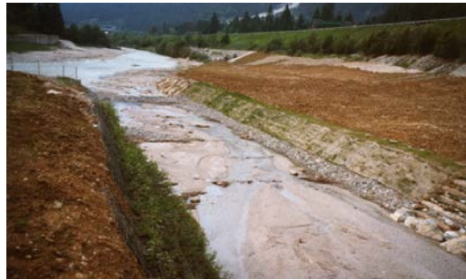
Fig. 2. Fella river confluence with the Saisera river; bank protection mattresses are visible, 2000
